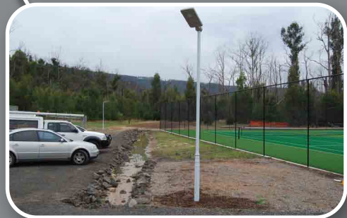
Rural & Remote Area Lighting
